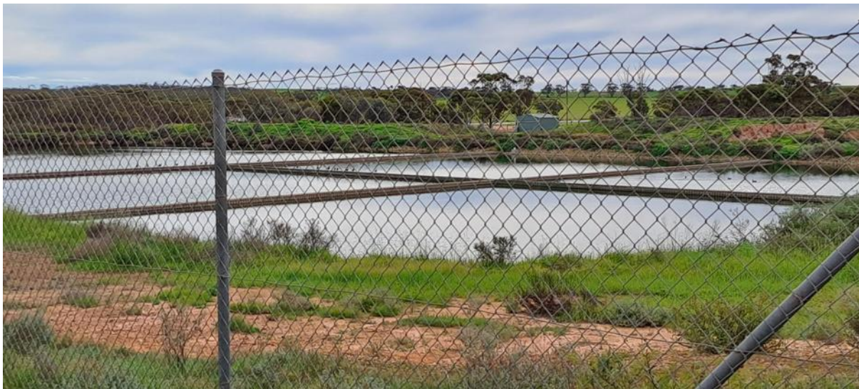
Facultative Lagoons in very good condition. Internal baffles exceptionally sound (unusual). Re-use Pump Shed in background.
