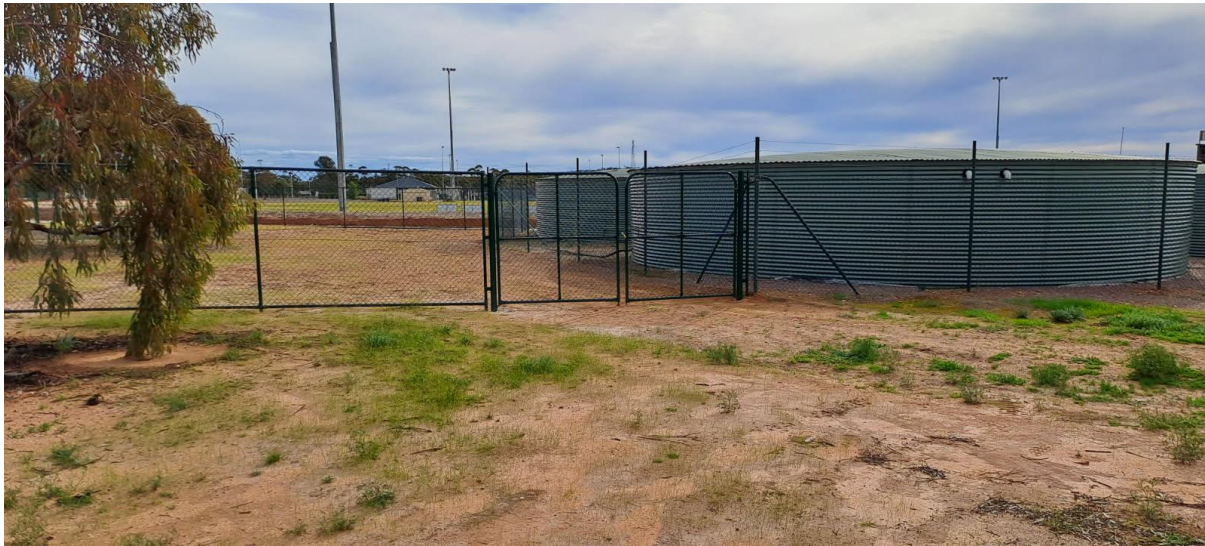
Buffer tanks at Football Oval. This IAMP terminates at the Tank Inlets.
